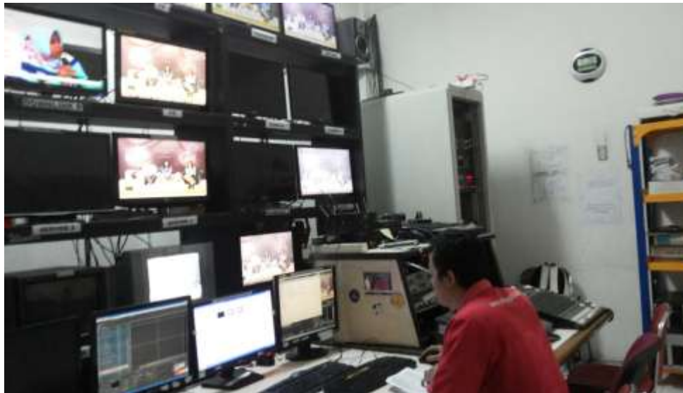
Master Control Room (MCR)
